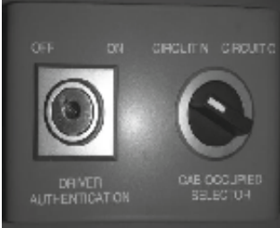
Cab Occupied Selector inside CRW Panel
